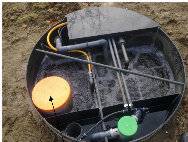
Chemical tank for phosphorous removal
